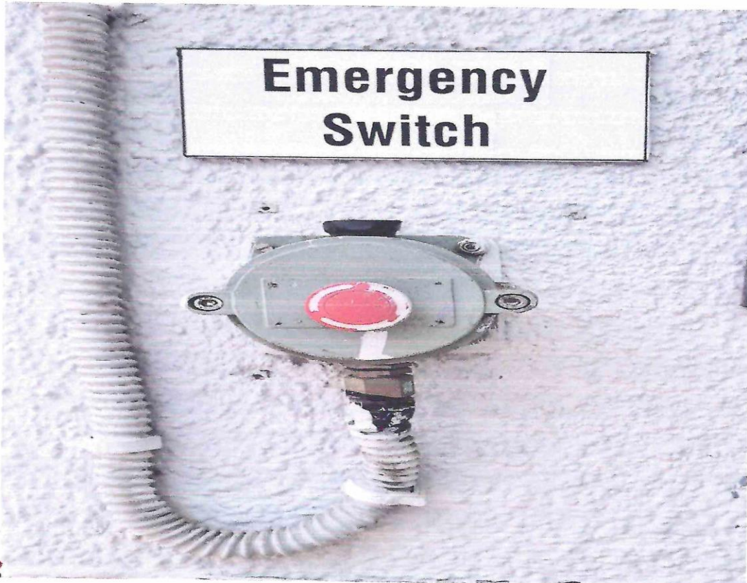
Fig: Emergency Stop Switch at the manufacturing plant
