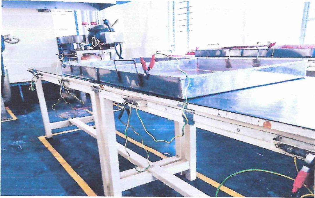
Fig: Trays & Working tables duly Earthed & Connected to Earthing Pit
