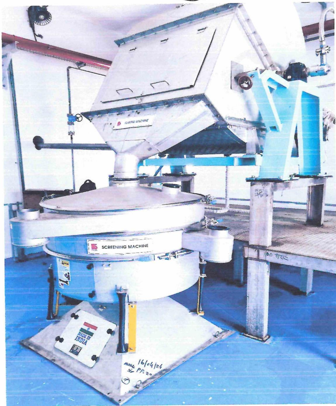
Fig: Screening Machine Installed at the TNT Manufacturing Plant
