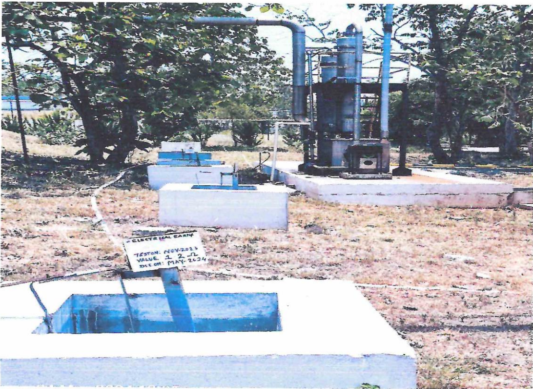
Fig: Earthing Pits and Fume Scrubbing System at HR CPCH Plant
