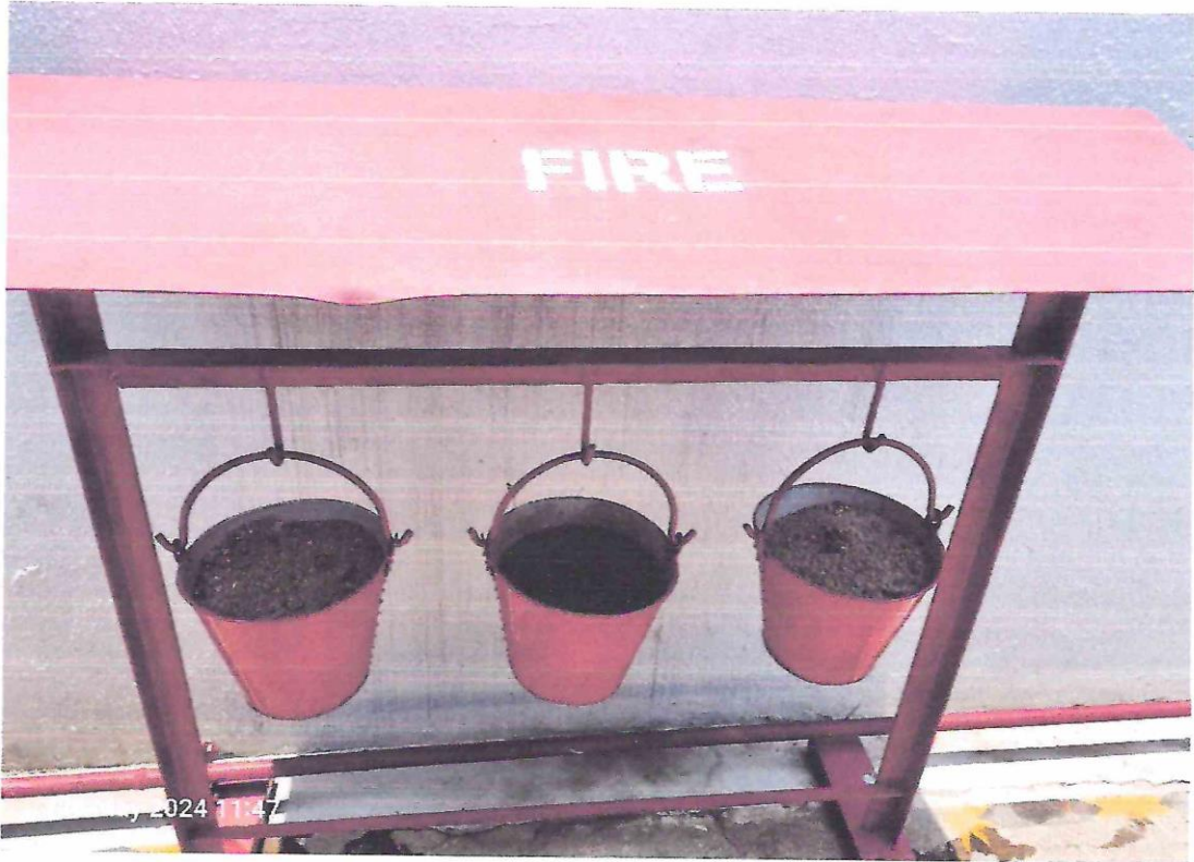
Fig: Fire Bucket filled with sand & water provided at the manufacturing plant
