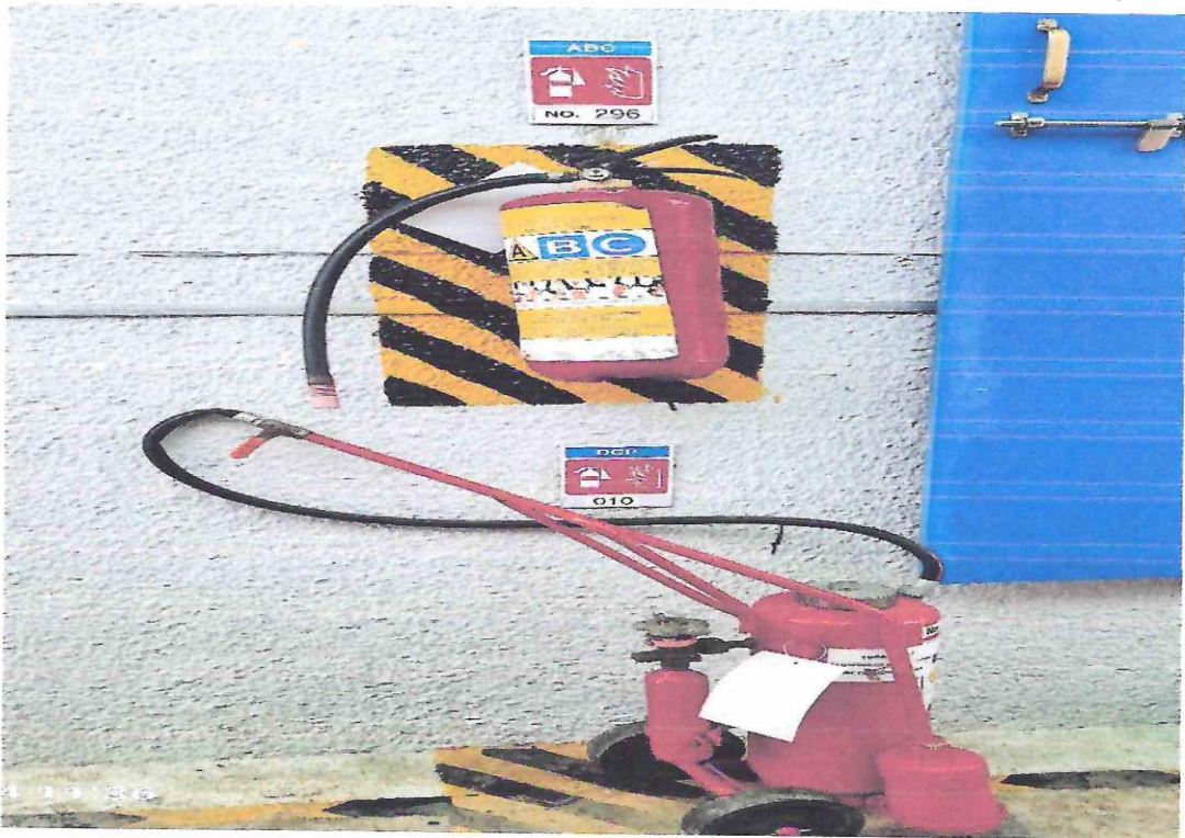
Fig: Fire Extinguisher provided at the manufacturing plant
